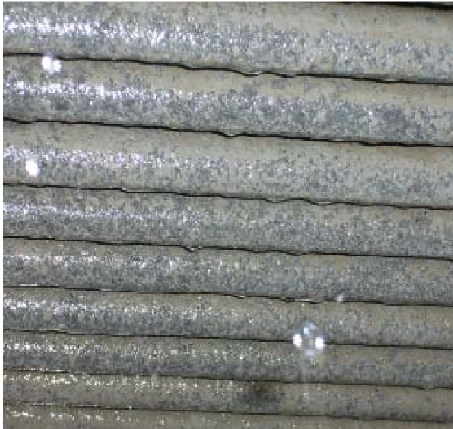
SCALE THICKNESS ON TUBES AFTER 75 DAYS OF INSTALLATION 0.05MM AT WORST PLACE
