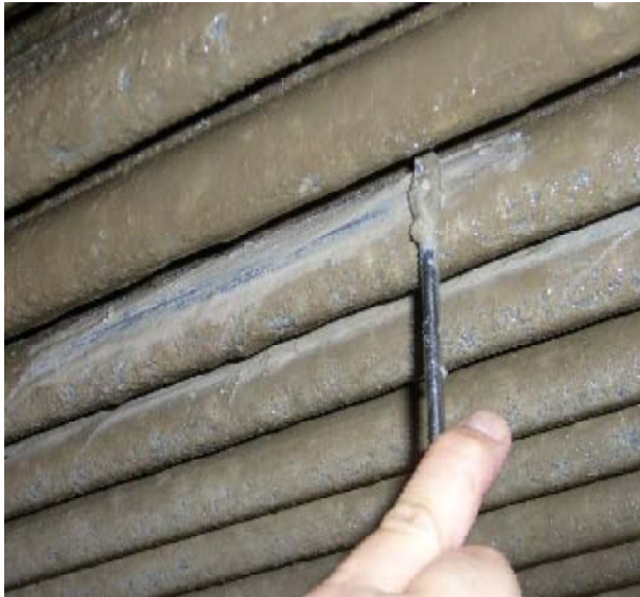
SCALE THICKNESS ON TUBES BEFORE INSTALLATION 2.00MM
