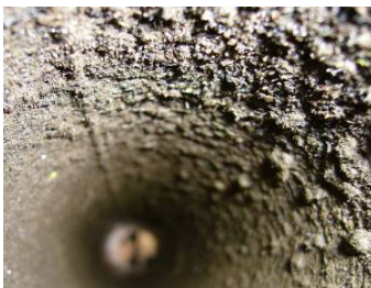
Above : Feed line to Compressors with scale deposition
