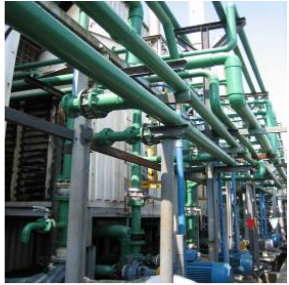
B-2 Water pump 22 Kw , 30 HP , pipe diameter is 4 inches. The water flow rate is 45 M3 / Hr. or Flow velocity is 1.54 m/ sec.
