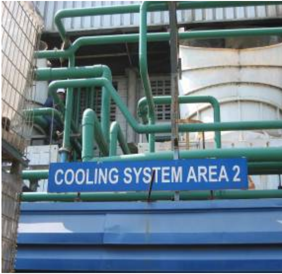
B-1 Location at CAT-100 installation
