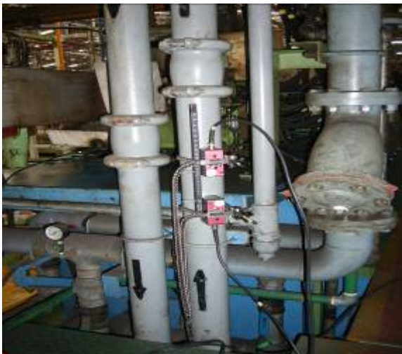
A-3 Flow Meter installed on the cool water inlet
